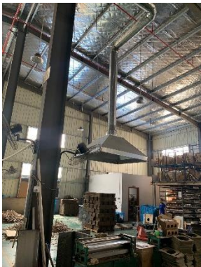
车间内废气集气罩
